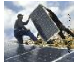
image BERLINER GEOSOL INSTALLING THE SOLAR ENERGY PLANT (PHOTOVOLTAIK) "LEIPZIGER LAND" OWNED BY SHELL SOLAR IN A FORMER BROWN COAL AREA NEAR LEIPZIG, SACHSEN, GERMANY.
