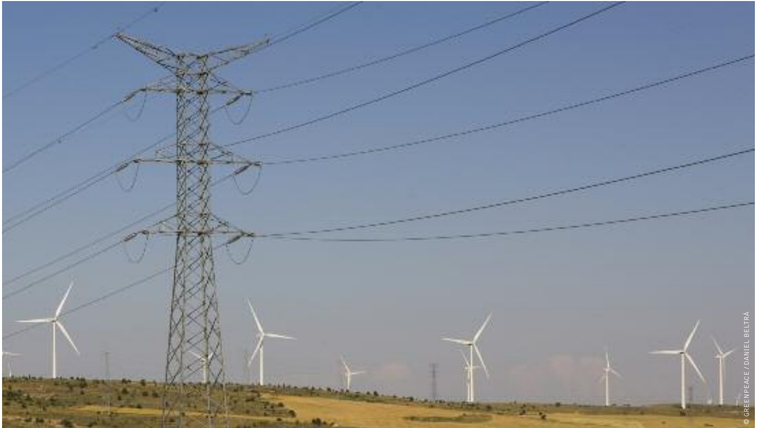
image THE MARANCHON WIND FARM IS THE LARGEST IN EUROPE WITH 104 GENERATORS WITH A TOTAL CAPACITY OF 208 MW, ENOUGH ANNUAL POWER FOR 590,000 PEOPLE. THE FARM ANNUALLY PRODUCES THE EQUIVALENT ELECTRICITY OF 100,000 TONS OF OIL, THEREBY ELIMINATING 430,000 TONS OF CO 2 .
