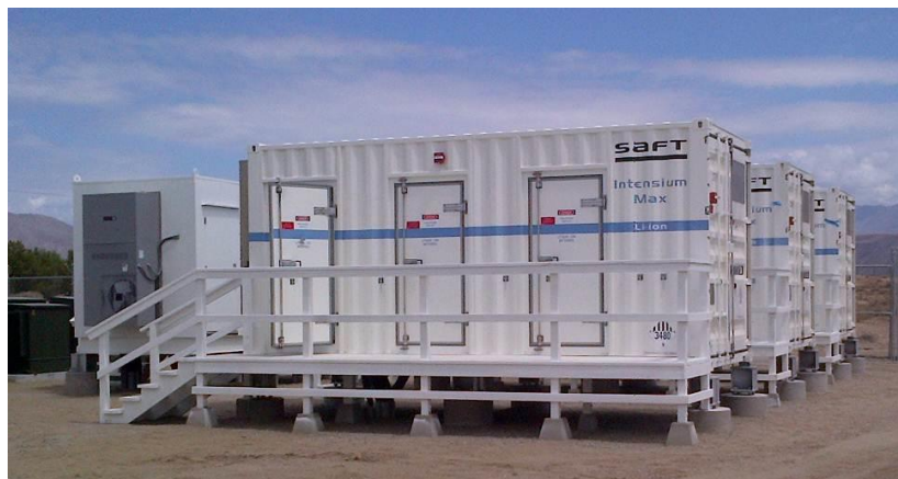
Figure 9: Advanced Energy Storage
