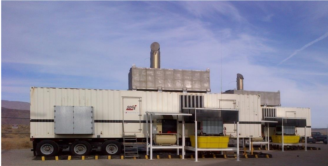
Figure 4: Microgrid Distributed Generators
