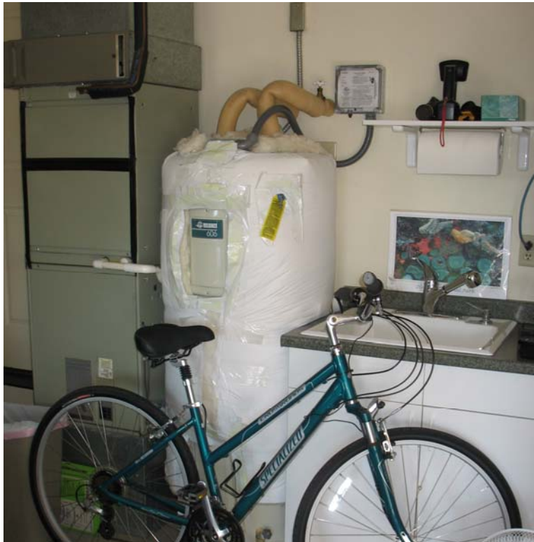
Figure 3.3. Load Control Module (LCM) and a Participant's Water Heater
