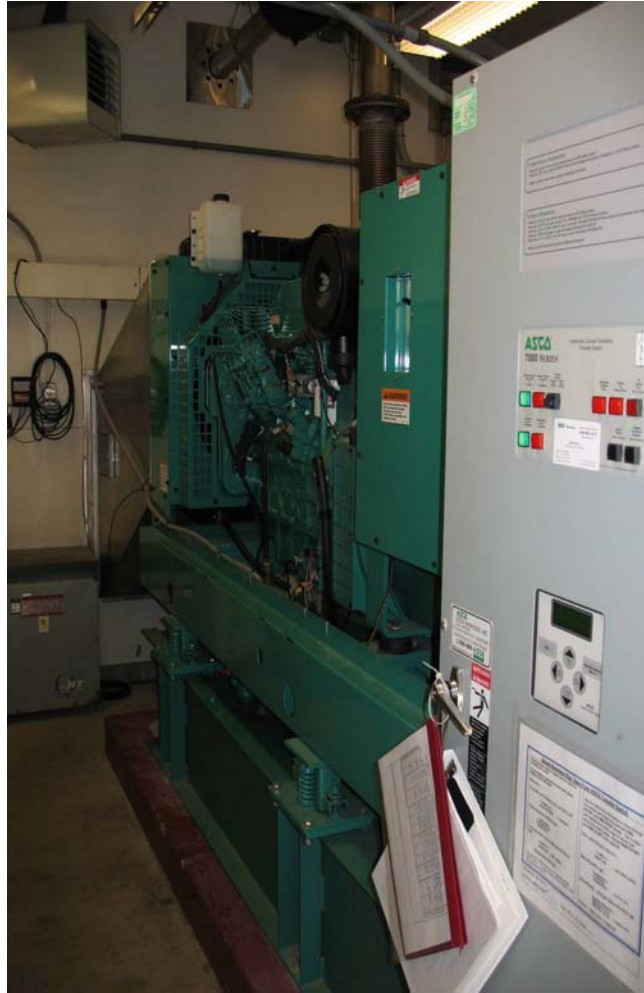
Figure 6.2. PNNL's 175-kW Kohler Generator and Automatic Transfer Switch
