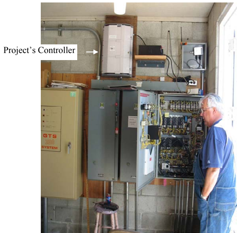
Figure 5.4. Control Panels at the Sekiu Pumping Station
