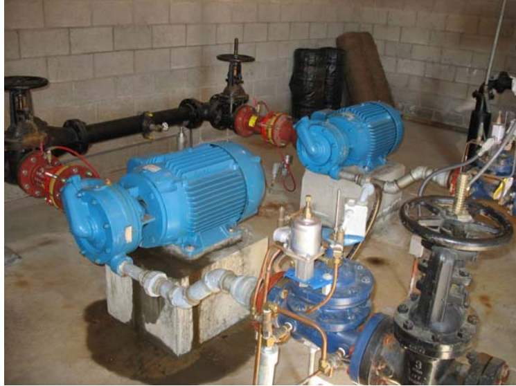
Figure 5.1. Pumps at the Sekiu Water Pumping Station
