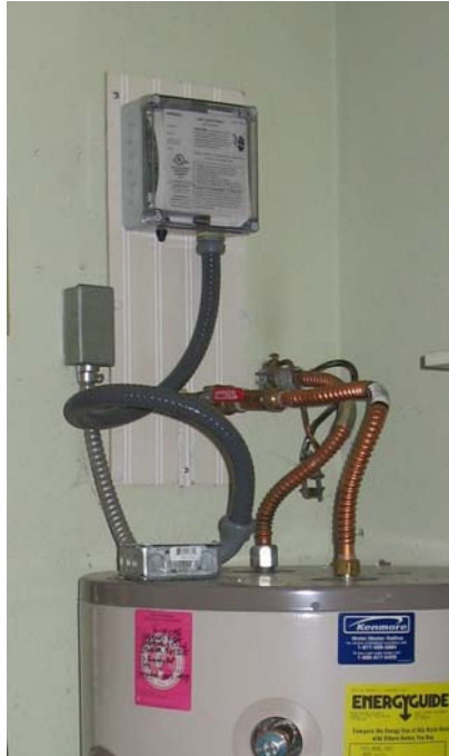
Figure 2.4. Load-Control Module Installed on Water Heater in a Project Home
