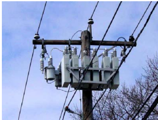
Automated Capacitor Bank
