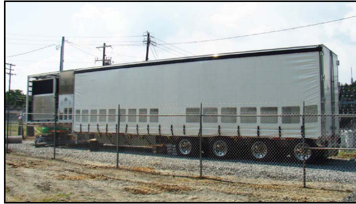
Figure 4-14 Premium Power’s 0.5-MW/2.8 MWh TransFlow 2000 Transportable Zinc-Bromine Energy Storage System, to be tested by EPRI and a utility consortium.
