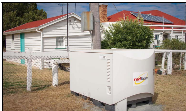
Figure 4-13 These 5-kW/20-kWh Community Energy Storage (CES) Systems by RedFlow Power and Ergon Energy of Australia will be linked by a Smart Grid network to provide megawatt-scale storage on the electricity grid.
