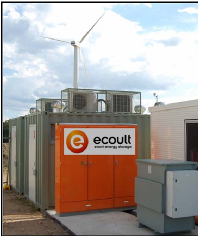
Figure 4-8 Phase 1 of Ecoult 1-MW/1-MWh UltraBattery system at Hampton Wind Smoothing Project in Australia (Source: Ecoult).
