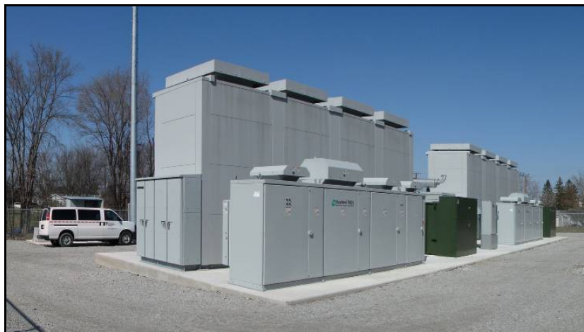
Figure 4-11 AEP Distribution Substation with Sodium-Sulfur Unit
