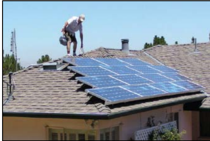
Figure 3-11 Residential Rooftop Photovoltaic Panels (Source: NREL)
