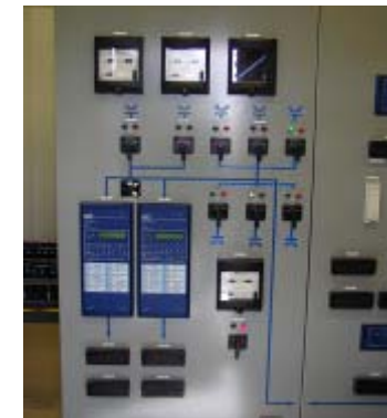
Sea West control panel (photo Steurer, Aug 2006)
