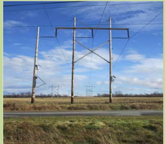
Figure 1. Dynamic Thermal Circuit Ratings provide real-time information about capacity in overhead transmission lines, like the one pictured below. Image courtesy of NYPA.
