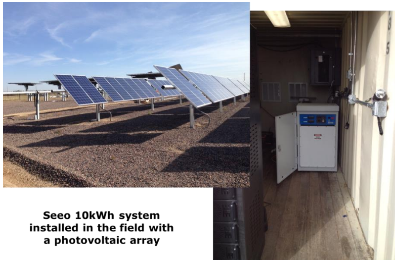
Figure 18: Field Installation of Seeo 10 kWh Energy Storage System
