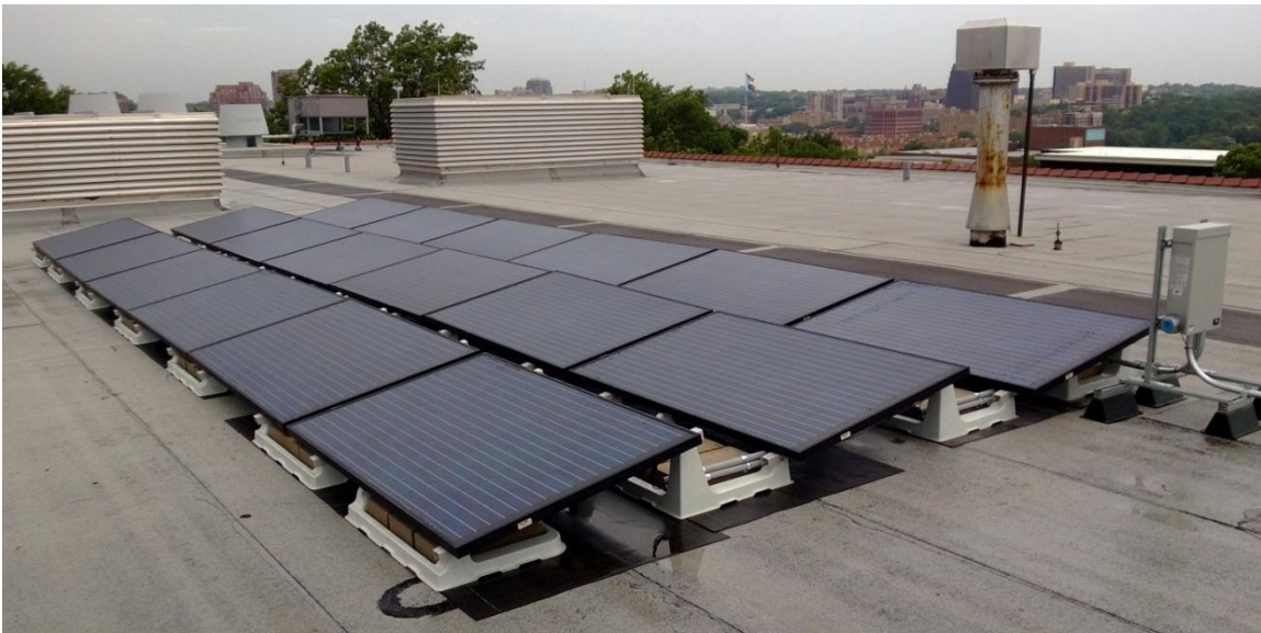
Figure 2-75: Typical Commercial PV Installation
