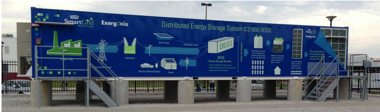
Figure 3-27: Battery Energy Storage System at SmartGrid Innovation Park
