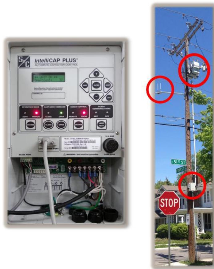
Figure 2-63: Typical Capacitor Bank Installation
