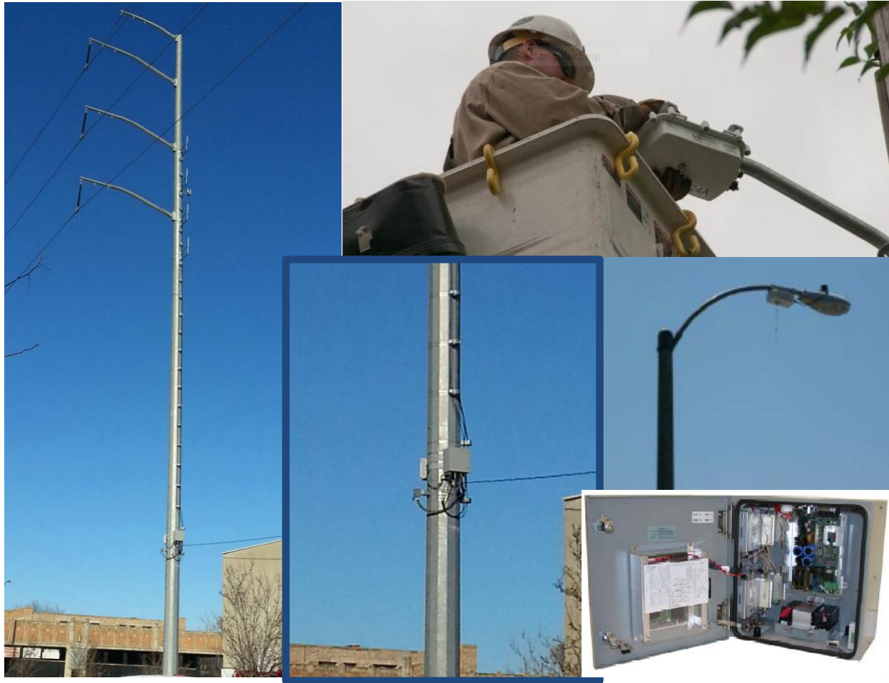
Figure 2-21 Installed AMI FAN Infrastructure
