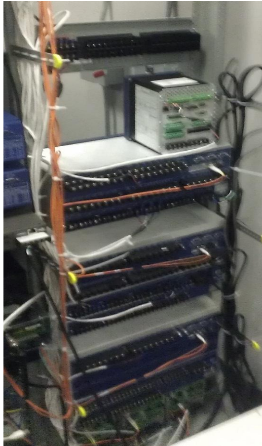
Figure 2-47: GOOSE Lab Testing Rack Setup
