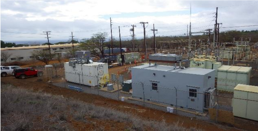
Figure 6-9: BESS installation in Wailea substation
