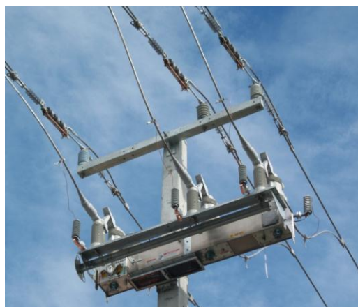
Figure 5. Automated Feeder Switches Installed by FPL.
