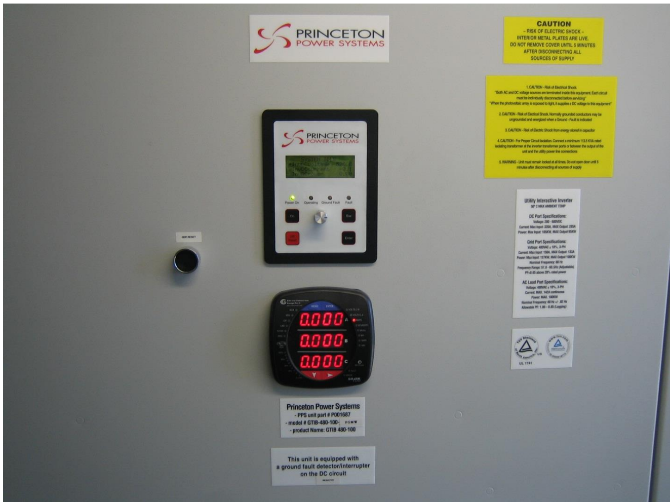
Figure 10 - Battery System Inverter
