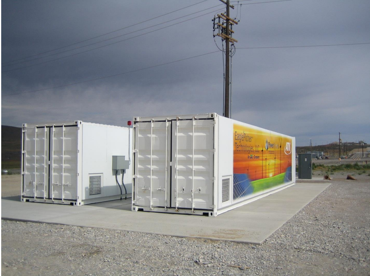
Figure 8 - 300KW Battery Storage System
