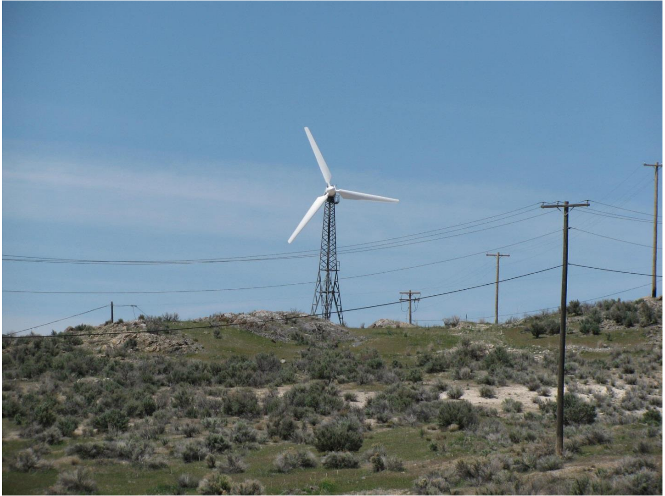
Figure 3 - Wind Generator in Operation
